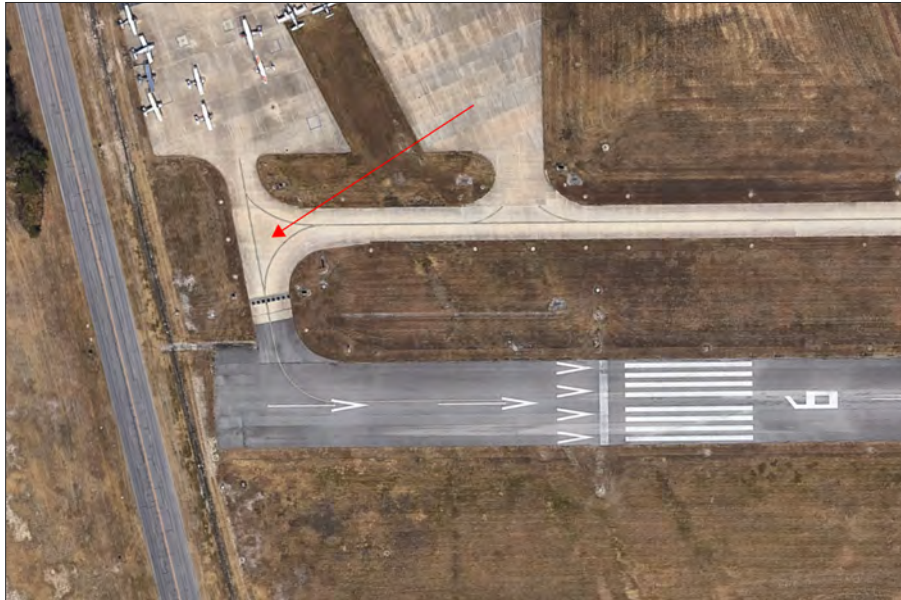
FIGURE 4-8 TAXIWAY CONFIGURATION DEFICIENCY STINSON MUNICIPAL AIRPORT
